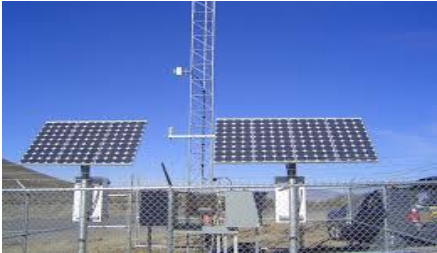
Images of rural broadband sector hubs, powered by solar electricity.
